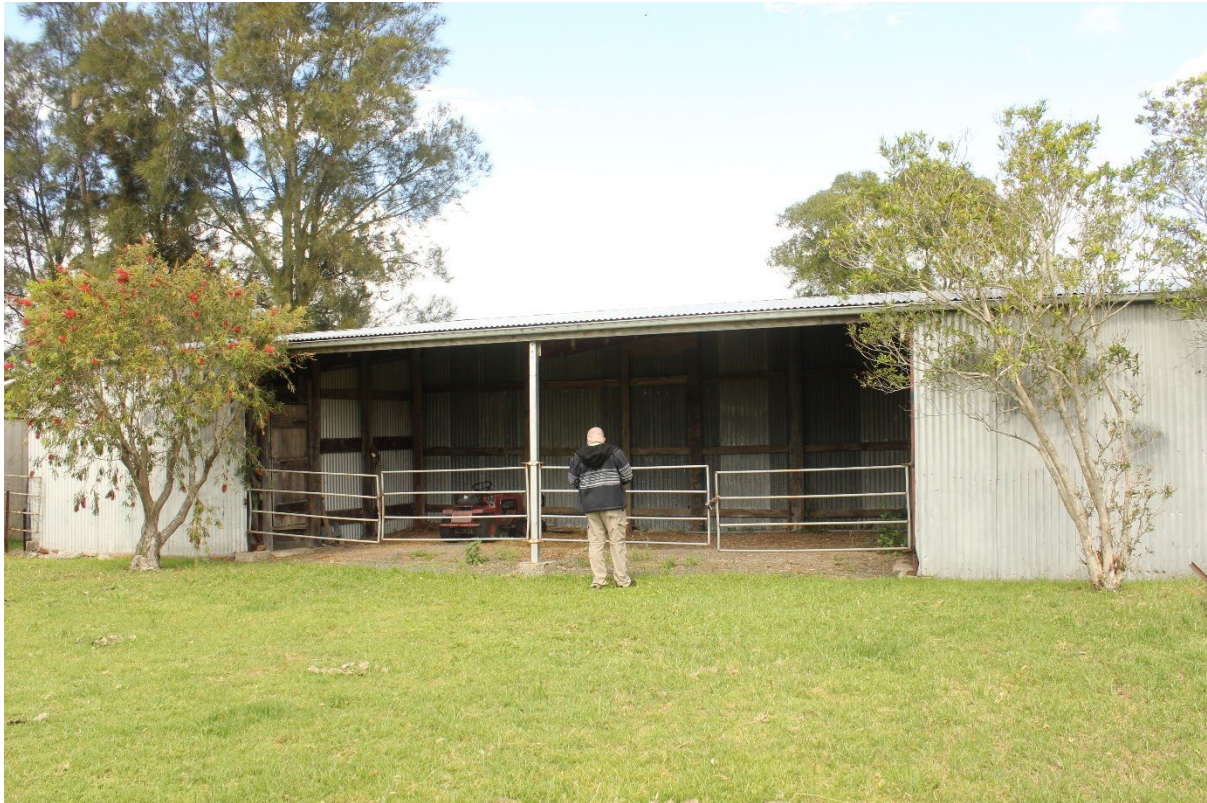
Figure 18: Showing detail of recent barn construction. The barn appears to have been constructed using recycled materials from an earlier barn of structure (as was indicated by Melinda on site).
